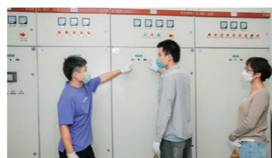
White glove inspection of power distribution room shows all-round unified high standard of precision work quality
